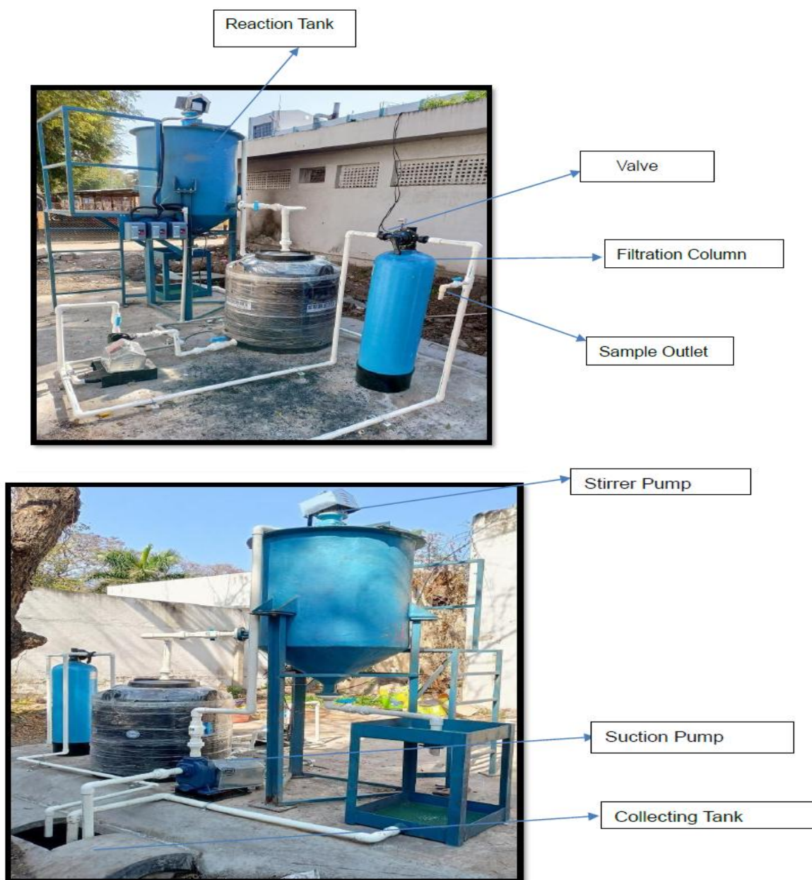
Figure: Effluent Treatment Plant
